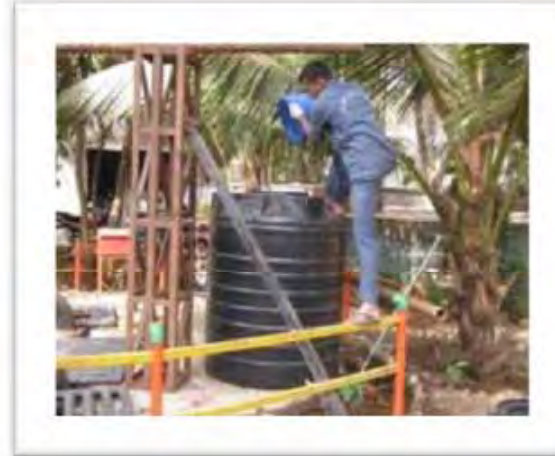
3. Dilution of concentrated Solution of Persnickety®713 in Dosing Tank in the ratio of 1:20 / 1:40 with Fresh Water or Treated Effluent from STP
